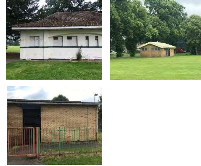
Existing Public toilets/Changing rooms in Pymmes Park, Craig Park, Florence Green park
