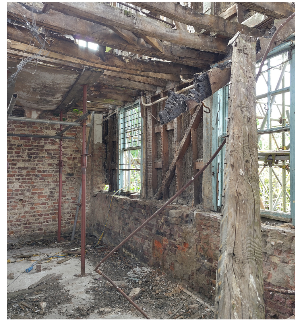
Above: Damage to the southwest corner of the building.
