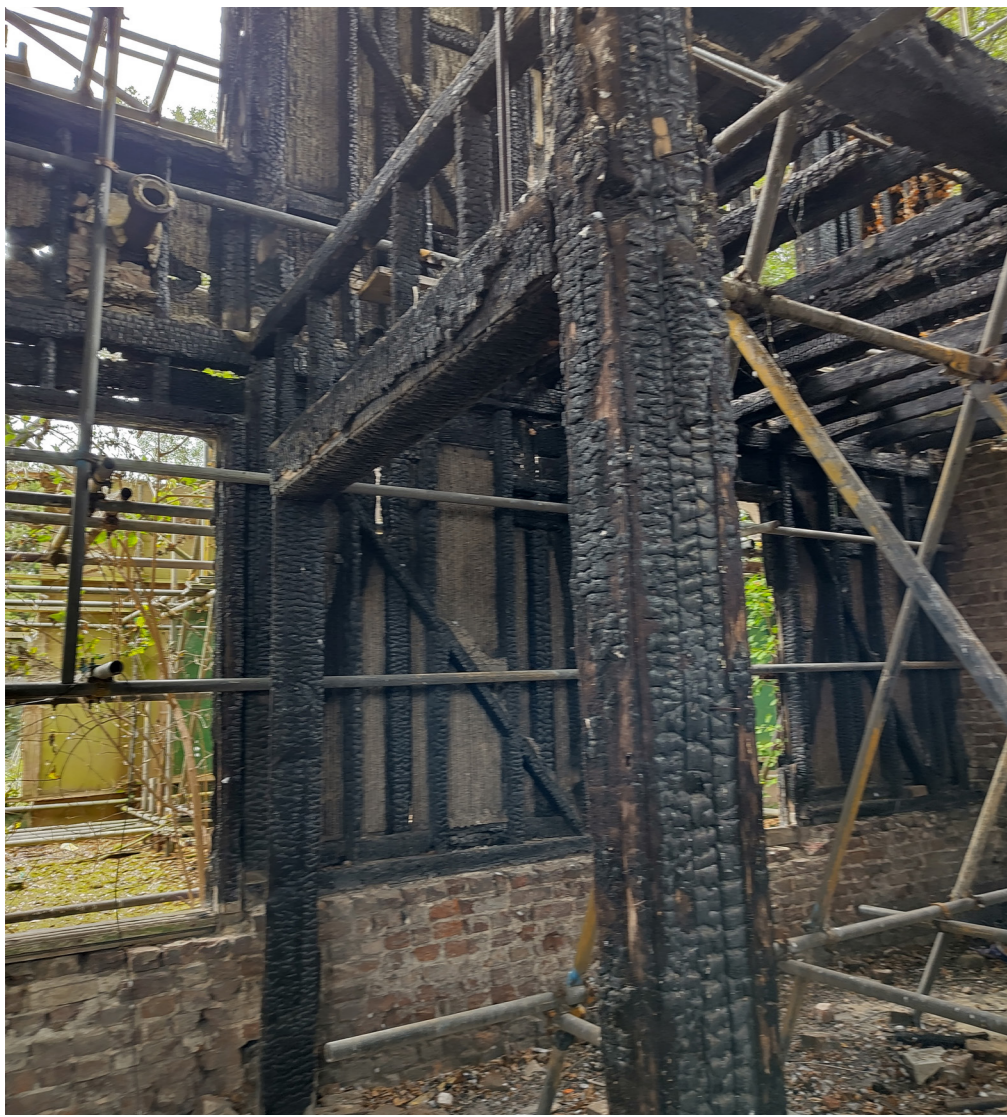
Above: Typical damage to the east elevation and first floor structure.
