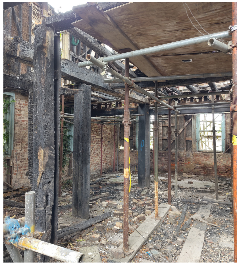
Above: Damage to structural timbers and first floor construction in the southwest corner.
