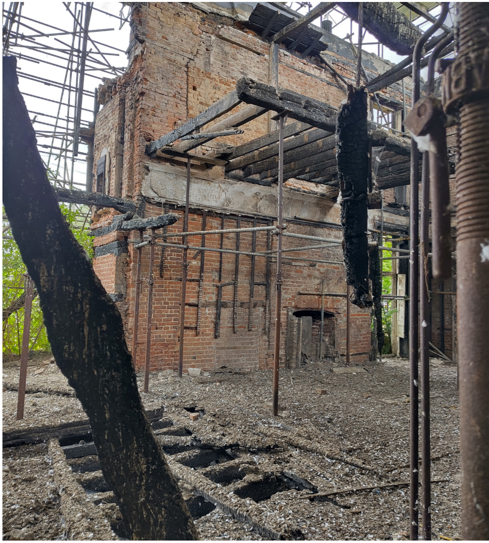
Above: The remaining first floor timber structure to the north of the building.
