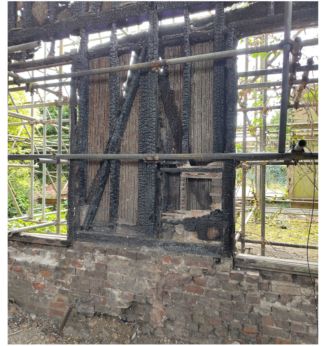
Above: Typical damage to the east elevation.
