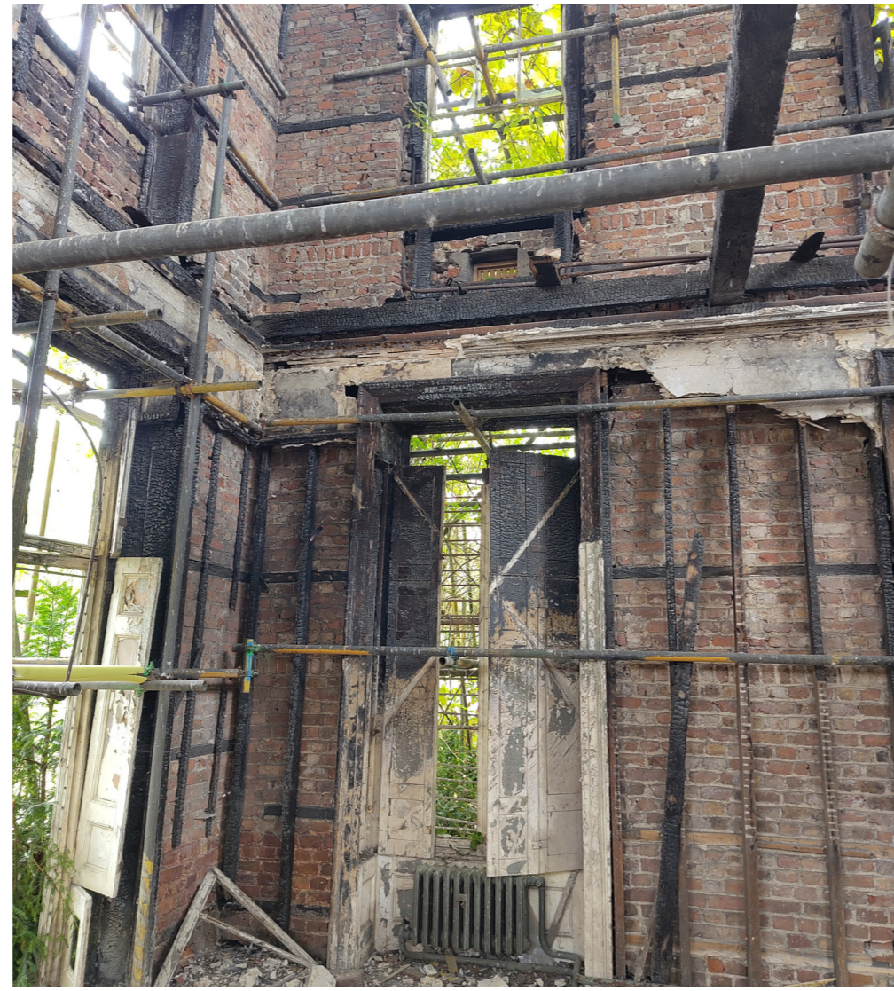
Above: Damage to the shutter and windows to the north elevation.
