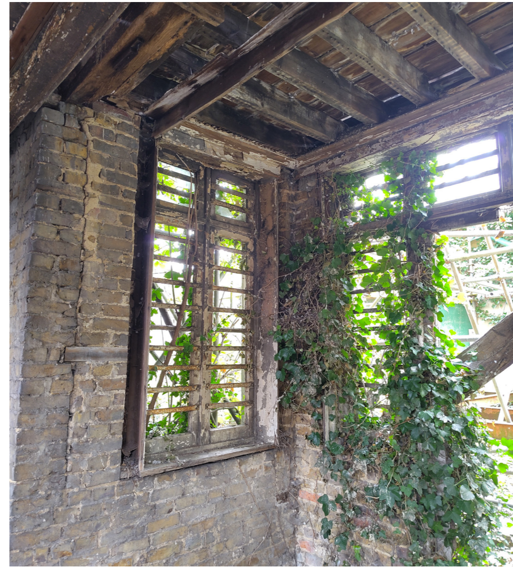
Above: Damage to the eastern porch.
