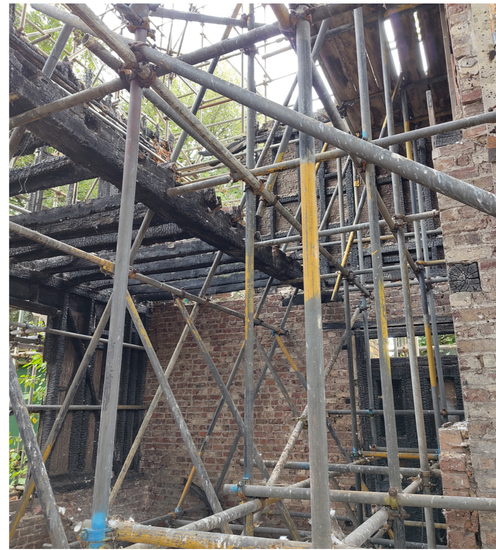
Above: Typical damage to the southern elevation.
