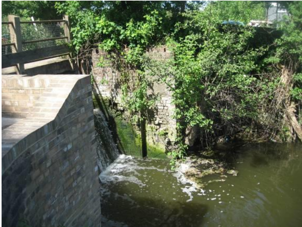
Figure 20: Weir walls in disrepair
