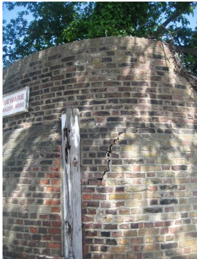
Figure 21: Cracks in boundary wall
