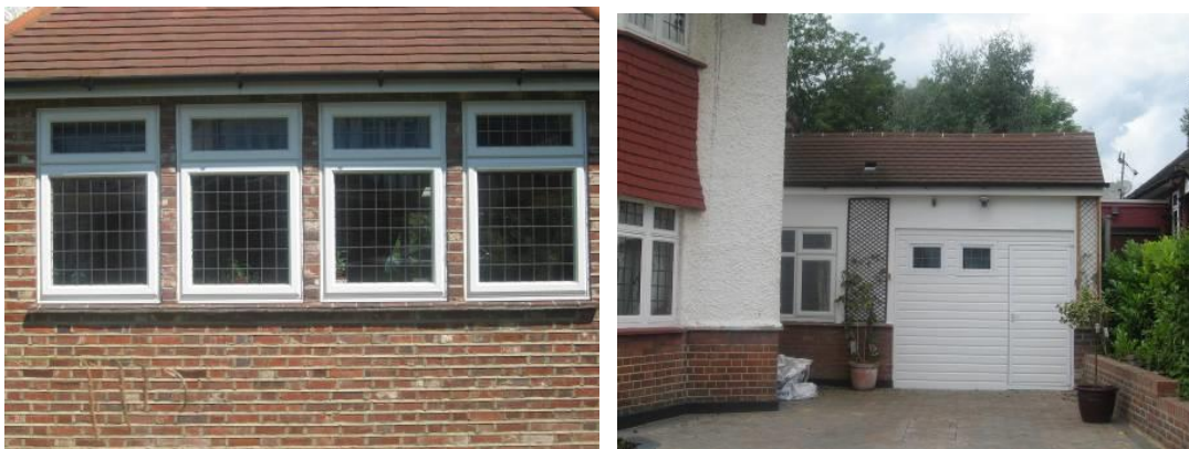
Figure 13: Inappropriate detailing to new work
